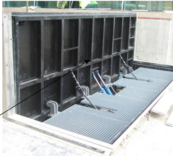
Example of flood barrier in Wakefield - Raised
