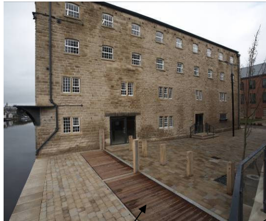
Flip-Up flood barrier in 'lowered/open' position
